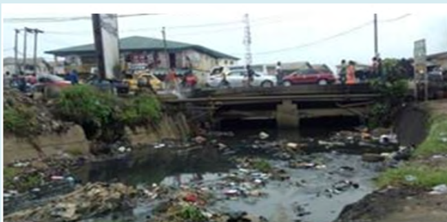
Figure 1: Wastes clogging stream channels at Ntawogba creek along Ikoku/Olu-Obasanjo Road.
